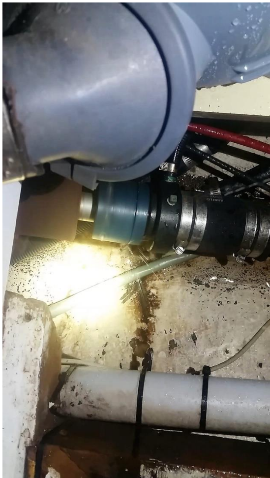
In case you were wondering what a leaking propeller shaft seal looks like
